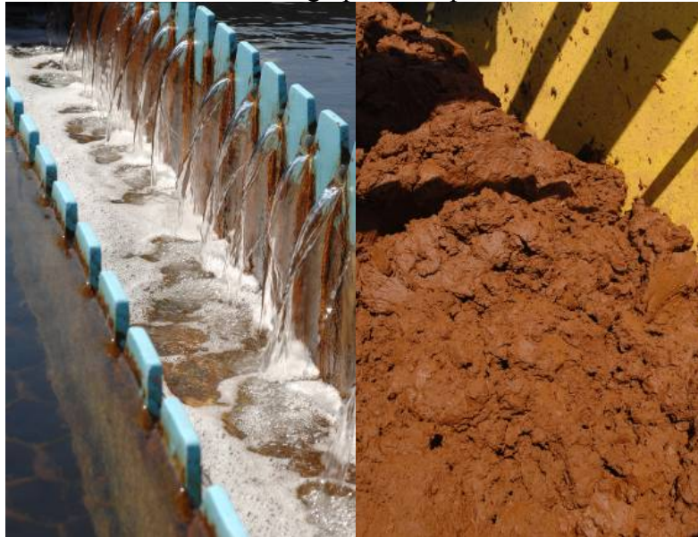
Figure's 9 and 10: 'Densadeg' – settling tank and typical sludge after being put through a centrifuge
